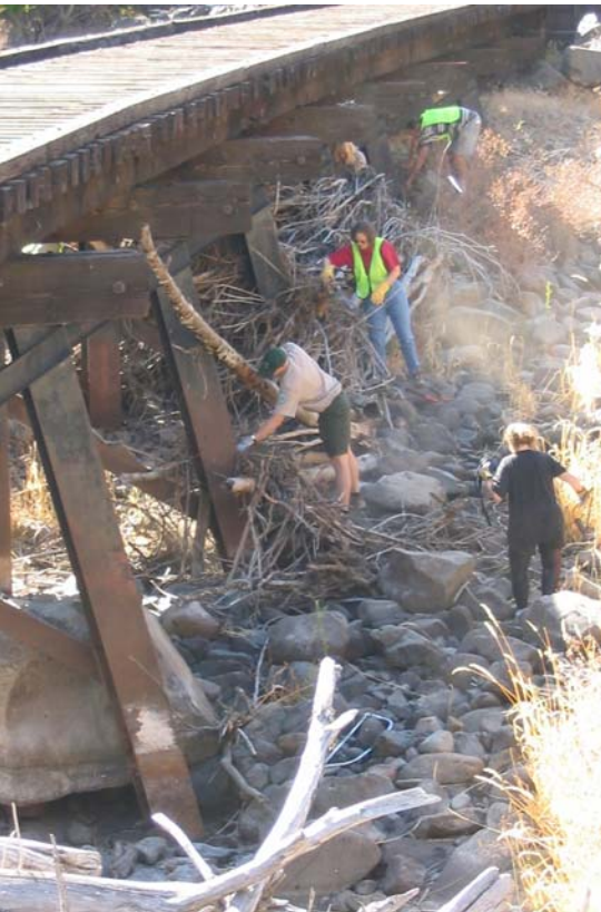
Volunteers remove tons of flood debris from a Swale Canyon railroad trestle. Pictured here in action are Andy Kallinan, Bev Linde and Donna Enz. Photo by Pam Essley
